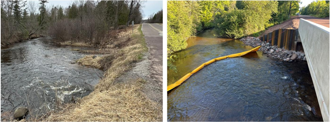
Figure 3 – The Choate Road crossing over Bluff Creek was improved to replace a set of culverts with a clear-span bridge. Shown above are the culverts (before) and the new bridge (after). This stream mitigation project was designed to improve fish passage and stream habitat quality. Additional restoration of in-stream features, both up and down-stream from the bridge, will be completed in September 2025.
