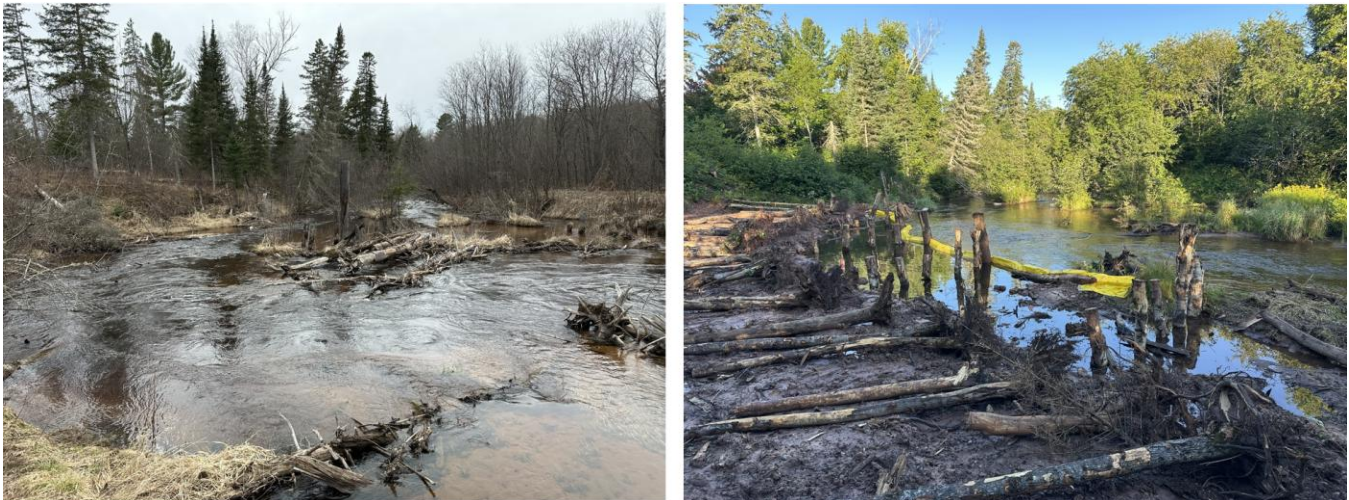
Figure 4 – Stream restoration in several sections of Bluff Creek is designed to improve stream flow properties and habitat quality. Shown above is a location where the eroded outside bank (left - April 2025) is in the process of being reconstructed (right - August 2025).
