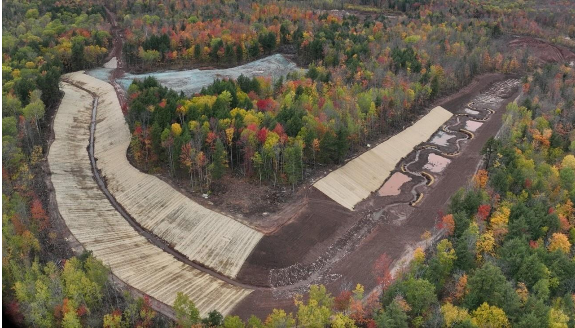
Stream diversion and mitigation: East stream diversion to divert water around future site infrastructure. Note the wetland mitigation construction within the stream diversion / mitigation area and the hydroseeded former wetland in the background.
